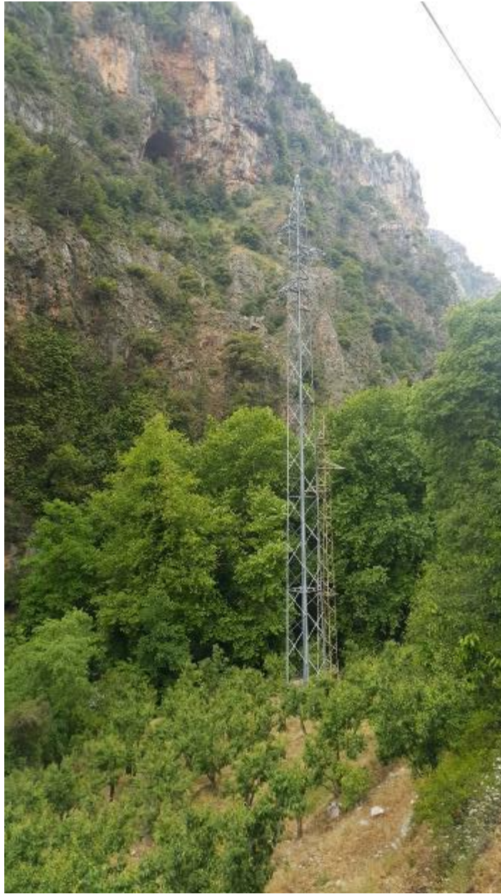
Figure 34. Towers of high voltage power lines in QV
